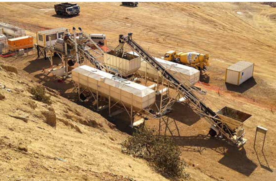
Planta de Concreto en Paita, Piura Concrete plant in Paita, Piura
